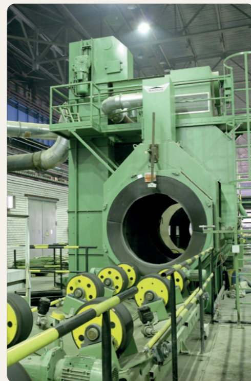
External Coating Plant
